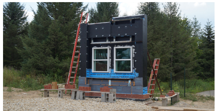
Materials testing mockup. To save on cost and time, smaller mockups of the envelope of a building will be produced to test various flashing, insulation materials, window installations and other variables to ensure proper function. Any issues are then resolved on a smaller scale prior to installation on an entire building. This particular mockup was rigorously tested for flashing installation, brick adherence and appearance, vapor barrier effectiveness and window sealant quality.
